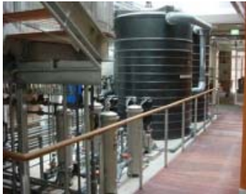
Recycle & Rainwater Treatment at 60L
